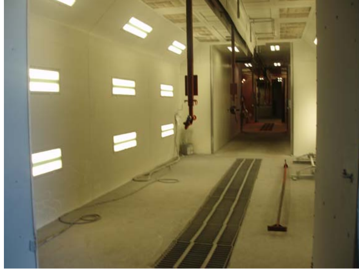
Monorail conveyor paint line (prime, paint and oven bake)
